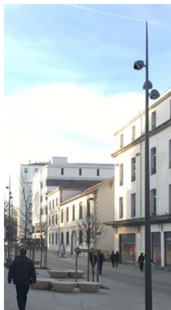
CCTV camera A dissuasive and visible solution, with an AXIS PTZ camera offering panoramic vision and the possibility of horizontal and vertical movement, allowing objects to be tracked on the move.
